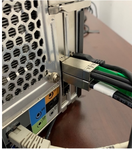
PCIe cables inserted into PCIe interface card's ports.
